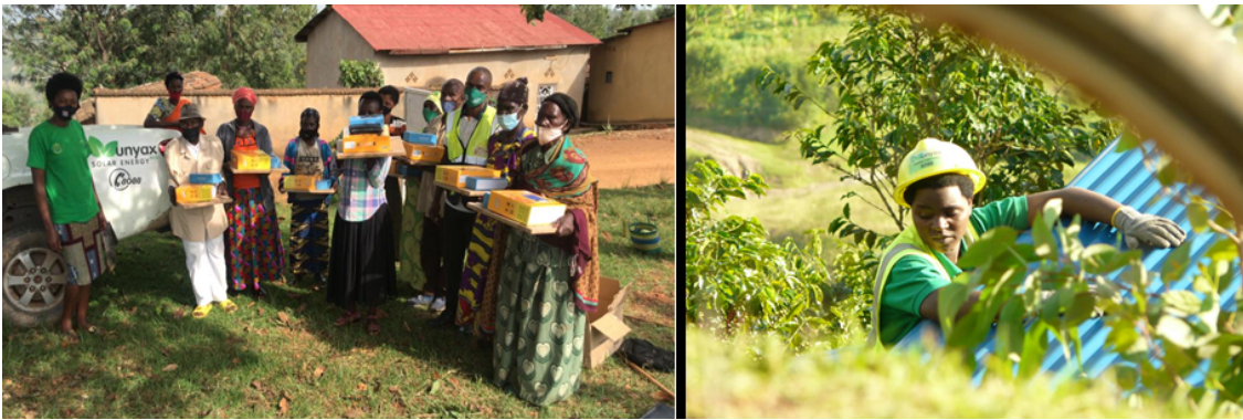
After SHS kits distribution, technicians go house to house to do installations
