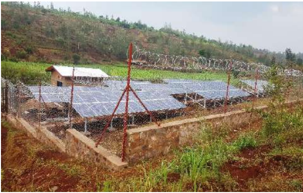
40 kWp Solar PV Mini-grid in Karusi- Burundi
