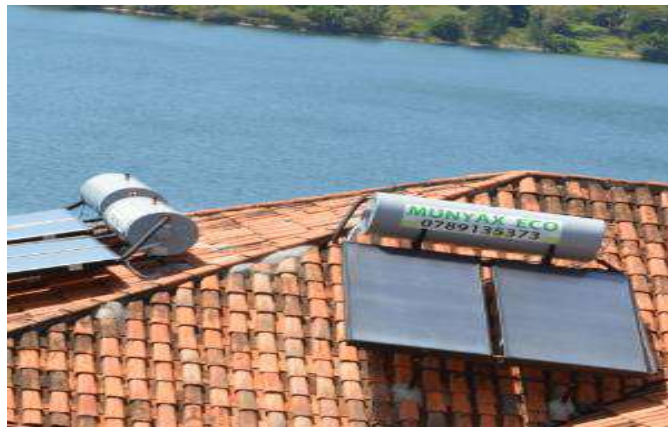
Solar water Heater at Bethanie Kibuye -Rwanda
