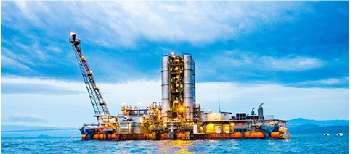
Photo: Kivu-Watt methane gas extraction facility
